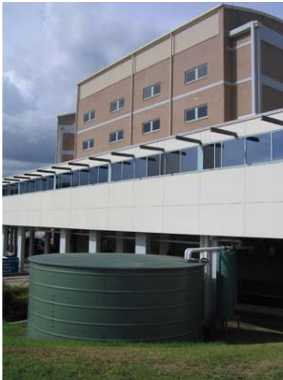
Rainwater Harvesting tank at hospital, Australia
