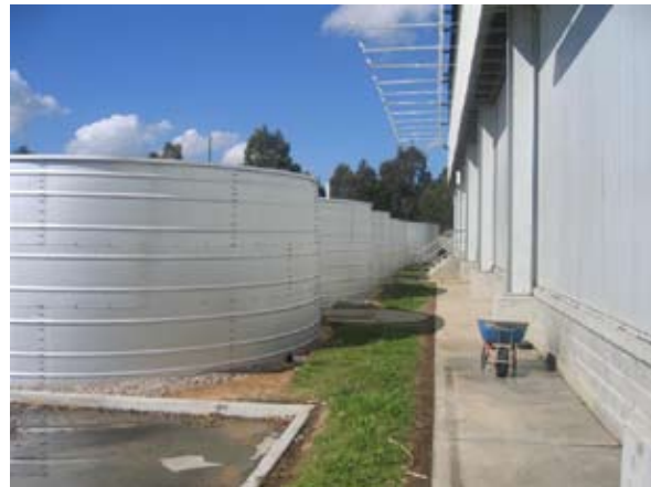
Commercial Rainwater Harvesting Woolworths RDC, Minchinbury, Sydney, Australia
